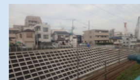
Slope after countermeasures (Senzokuike Station to Ishikawadai Station on the Ikegami Line)
