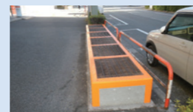
Raising of ventilation openings (Between Sangen-jaya Station and Sakurashinmachi Station on the Den-en-toshi Line)
