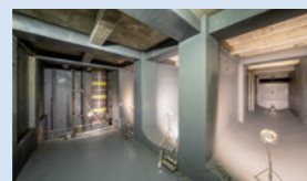
Rainwater harvesting facility at the east exit of Shibuya Station
