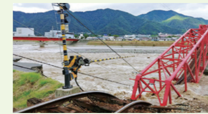
Bridge along the Ueda Dentetsu Bessho Line over Chikuma River collapses
