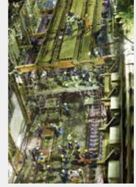
Converted from above-ground to subway line in one night, beginning interaction of the Toyoko and Fukutoshin Lines
