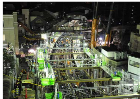
Transfer railroad track to the underground rails from Shibuya sta. to Daikanyama sta.
