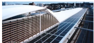
Solar panels at Motosumiyoshi Station
