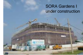
A panoramic view of Binh Duong New City (The Administration Center under construction)
